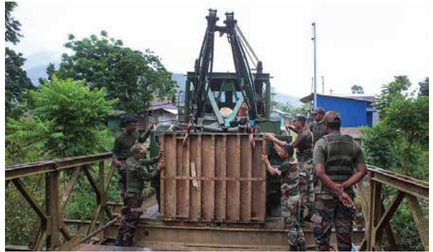
Road to recovery: Army jawans repair a damaged bridge at Leitanpokpi in violence-hit Manipur. PTI
